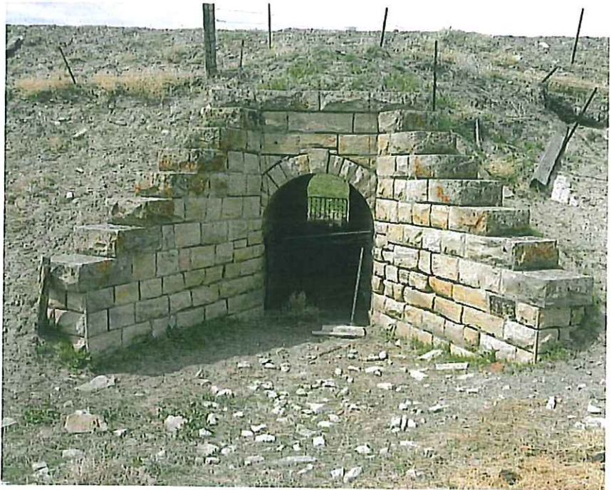
Above: Culvert 759, located three miles east of Harrison, served a dual role as a drainage structure and a cattle underpass. It was built in 1901 with a 6-foot opening. — Jerry Penry photo
