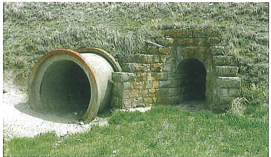
Below: Culvert 767, built in 1901 with a 48-inch opening, later had an 84-inch concrete pipe added next to it. It is located 1.5 miles west of Harrison. — Jerry Penry photo
