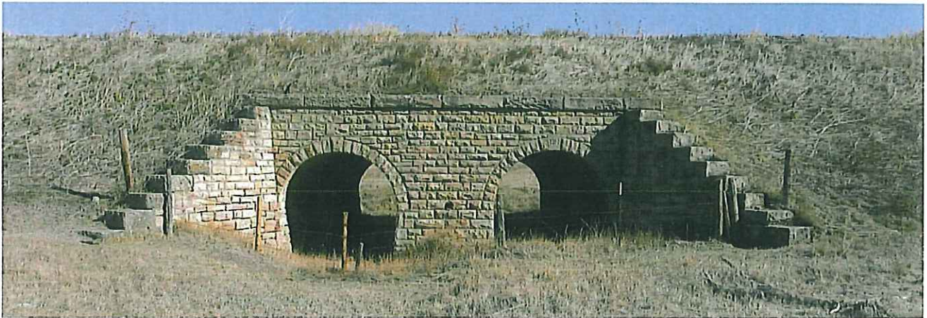
Above: Culvert 622 is a twin 10-foot structure that was built in 1898 and rebuilt in 1911. One of the original wingwalls had to be moved. — Jerry Penry photo
