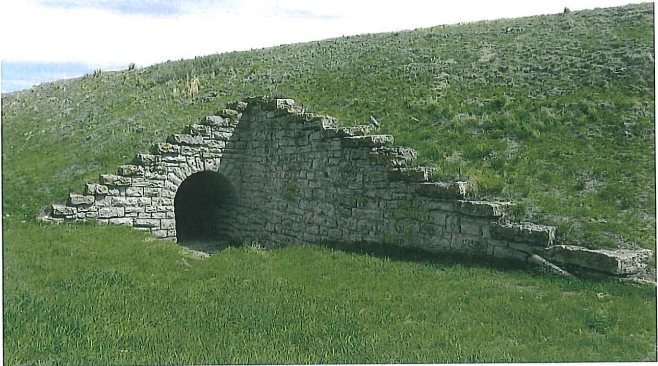
Above: Culvert 758 6/9 is constructed of poor grade native limestone from the area located 3.5 miles east of Harrison. It was built beneath a 2-degree curve in 1896. This impressive structure has a 9-foot opening and is 202 feet long with extended wingwalls. — Jerry Penry photo
