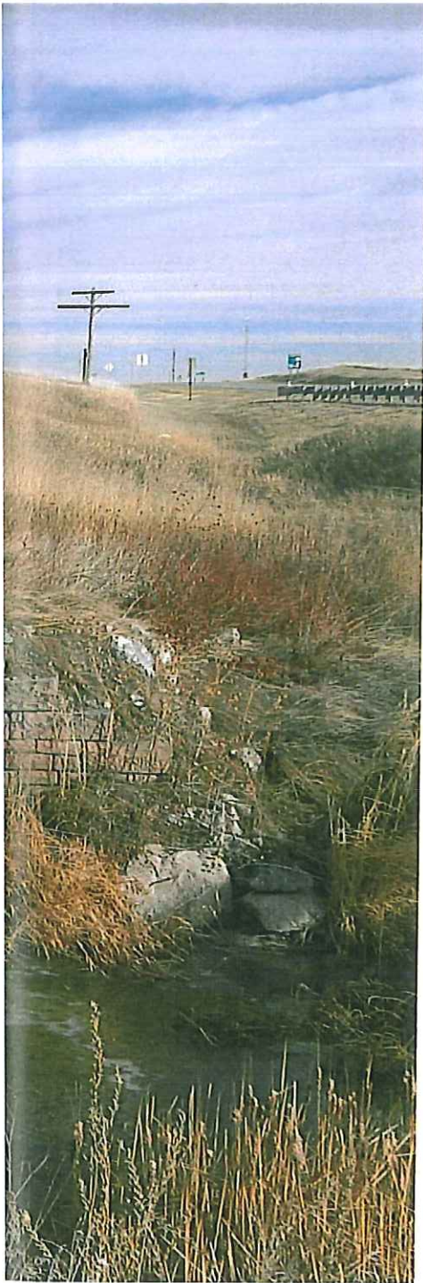
Opposite page left and right: Culvert 653, located three miles east of Chadron, was originally built as a single 10-foot opening in 1898. In 1911, a matching culvert was built next to it with the new stones woven into the earlier structure. The opposite page lower right image shows Pile Bridge 654 as it overwhelms the earlier stone arch culvert built at this location east of Chadron. — Jerry Penry photos
