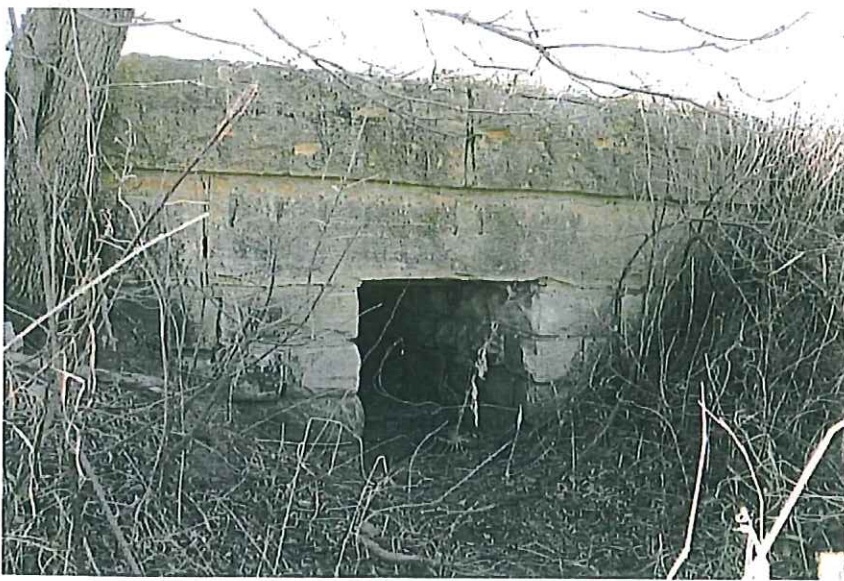
Above: Culvert 316 near Emmet is a 3-foot x 3-foot stone box which represents the simpler and more widespread method of making a culvert by a crew not skilled in the fine art of making a stone arch. —Jerry Penry photo
