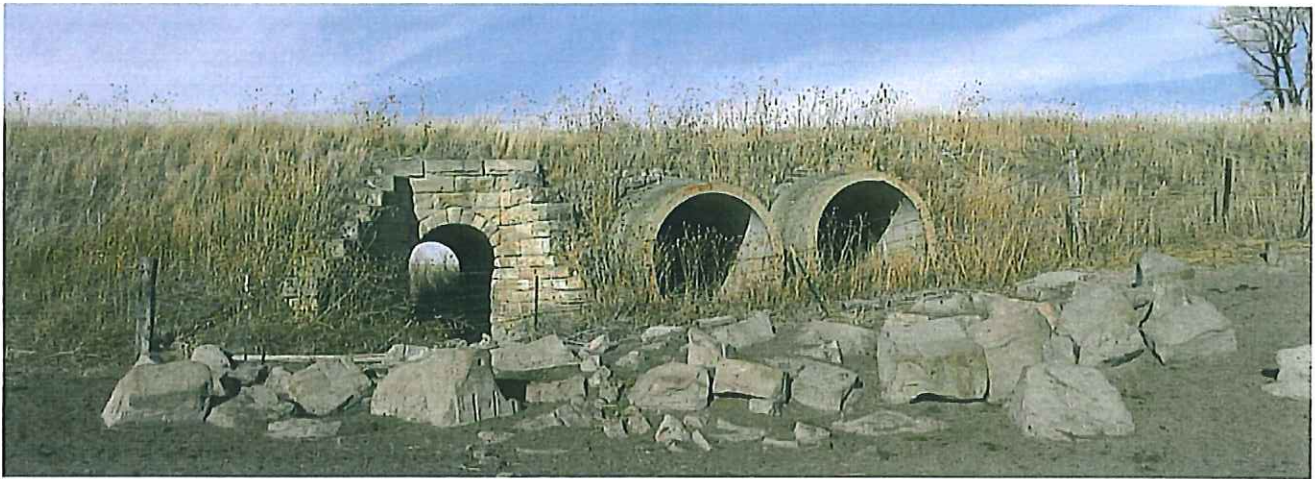
Above: Culvert 552, located five miles east of Gordon, was later assisted with two 84-inch concrete pipes to handle more drainage. — Jerry Penry photo
