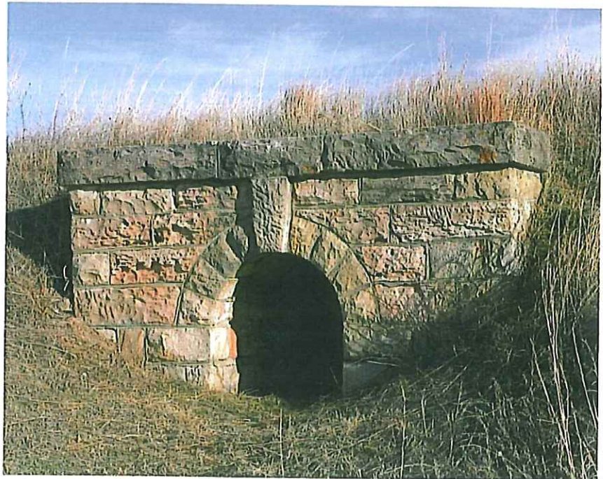
Above: The last stone arch culvert heading east on the Cowboy Line is No. 337 2/5 located three miles west of Atkinson. It was built in 1907 with a 54-inch opening. — Jerry Penry photo
