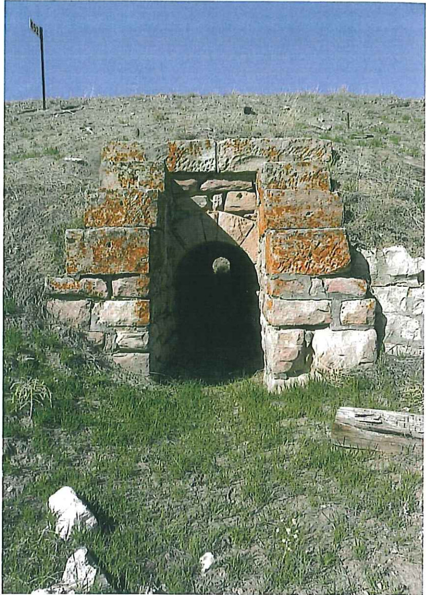
Above: Culvert 753 has a 36-inch opening and was built in 1896. It is located at milepost 452 just west of the former station of Andrews. — Jerry Penry photo
