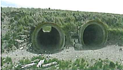
Above: The ends of Culvert 768 west of Harrison had concrete pipes added to the openings. — Jerry Penry photo
