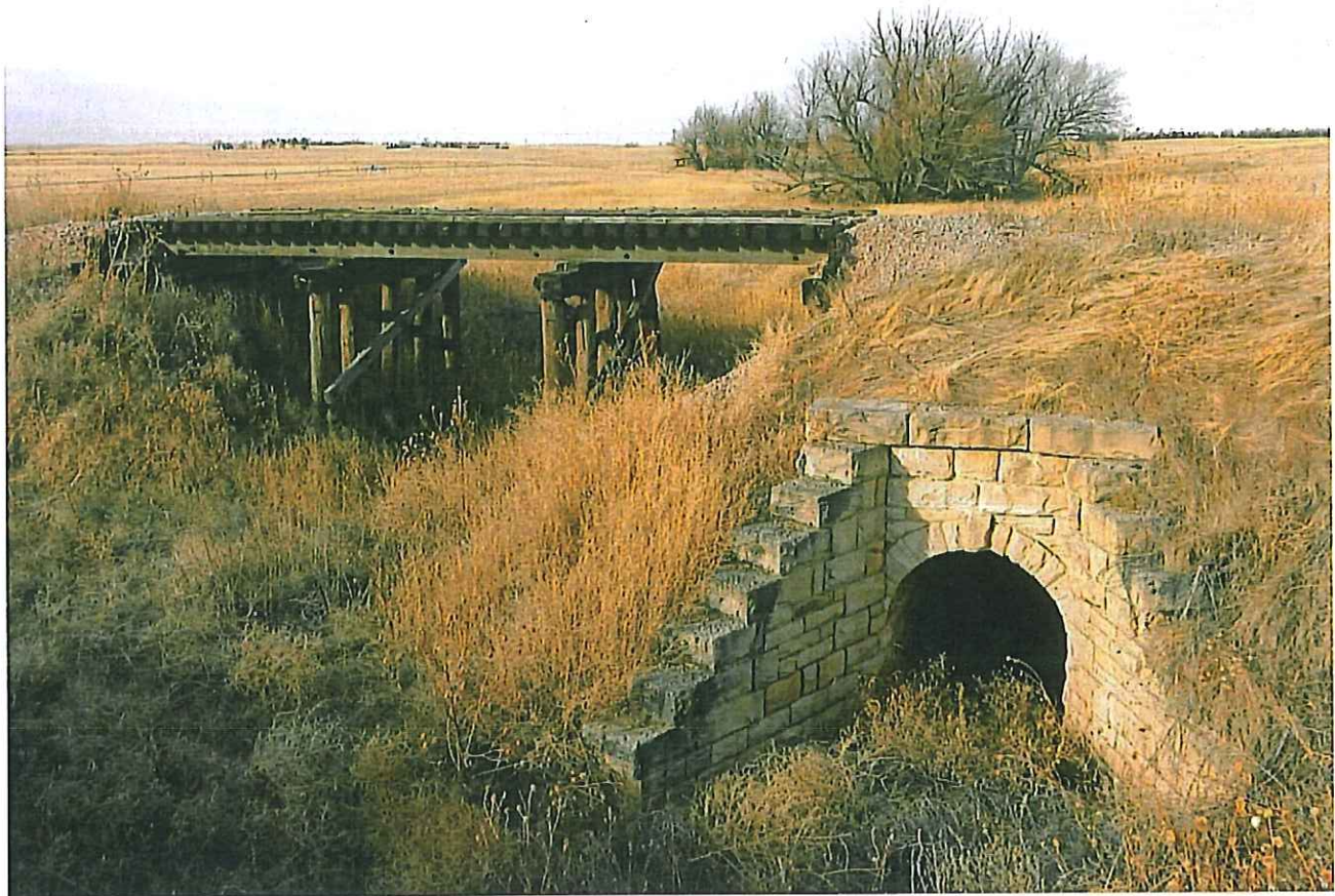
Above: Culvert 596 3/4 has a 6-foot opening but was built too small to handle the drainage. A three-span pile bridge was later built alongside. The culvert is located five miles west of Rushville. The culvert and bridge are similar to Culvert 654 and its bridge. — Jerry Penry photo
