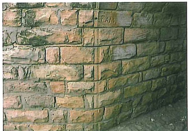
Above: The intricate masonry work by Berg and his crew can be seen where the tight-fitting stones of the wingwall meet the straight section of Culvert 578. — Jerry Penry photo
