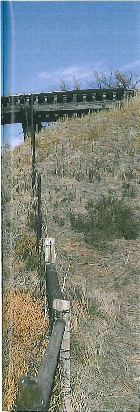
Above: Culvert 654 is located 2.5 miles east of Chadron. The 48-inch opening was later determined to be insufficient, so a six-span pile bridge was built adjacent to it. — Jerry Penry photo
